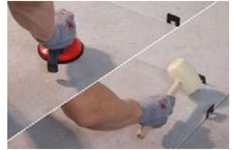
12- Both during installation and at the end of the day, check the quality of the work carried out before the bonding material sets. Correct any defects using suction cups and rubber mallets.
